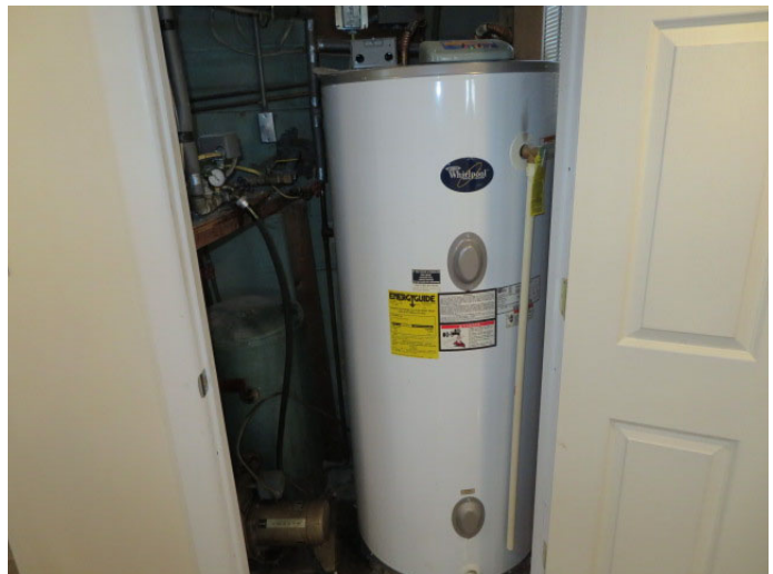
Water heater and well pump equipment.
