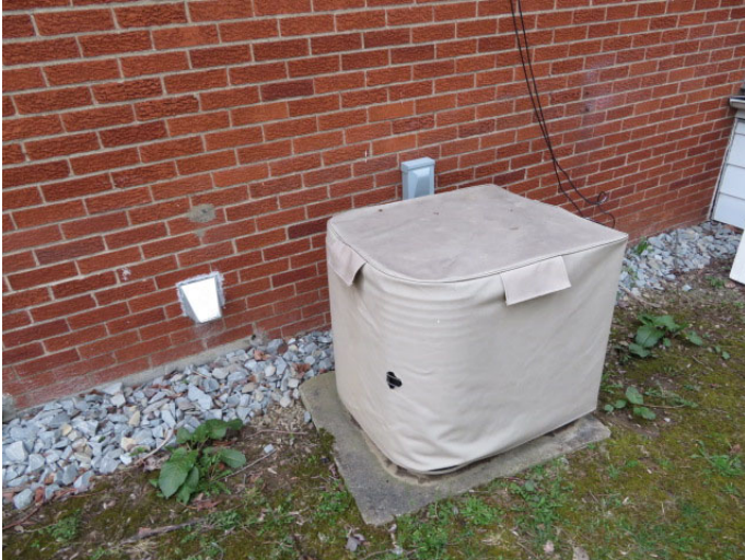
A/C Unit. The A/C unit should also undergo routine service to ensure that it is in full working order.
