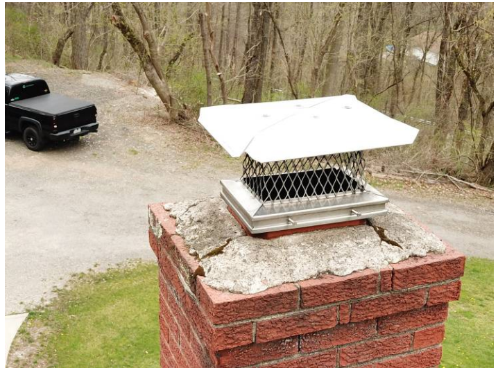
Basement fireplace chimney. It is recommended that both chimneys be evaluated by a qualified masonry or chimney contractor. The cement chimney caps are deteriorating. This can lead to water intrusion and damage to the bricks.
