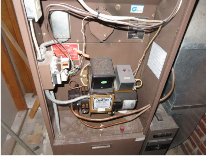
Oil furnace. It is recommended the furnace be serviced by a qualified HVAC technician to maximize its economic life.
