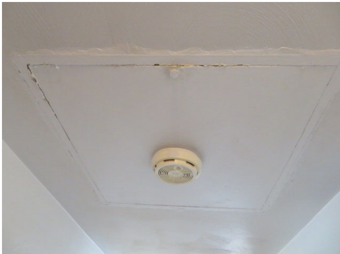
The attic hatch was nailed and painted shut making the attic inaccessible at the time of the inspection.
