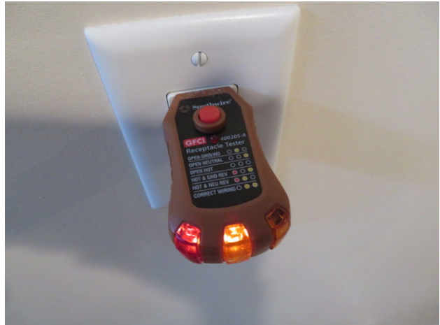
Hot/ neutral reverse receptacle in the basement laundry area.
