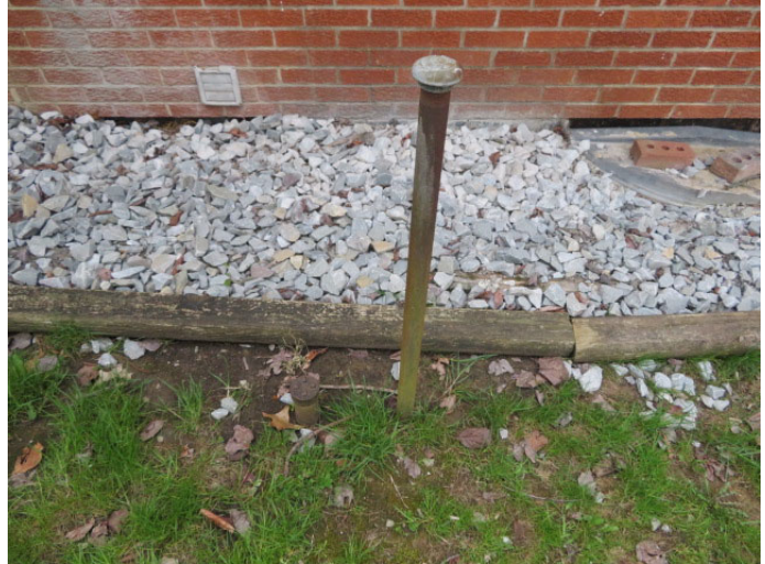
Underground oil tank fill tubes.
