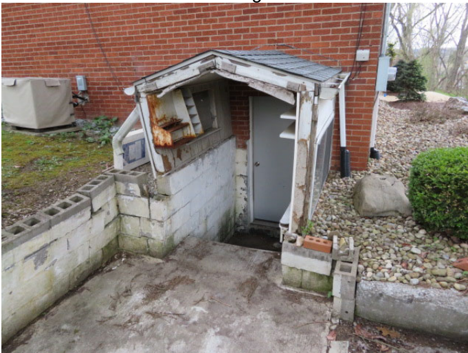
Walk out basement door. The retaining walls and roof around this entrance are in need of maintenance or repair.
