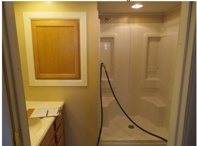
The light in the basement bathroom shower should have a water resistant cover installed prior to use of the shower.
