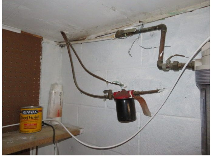
Furnace oil supply filter.
