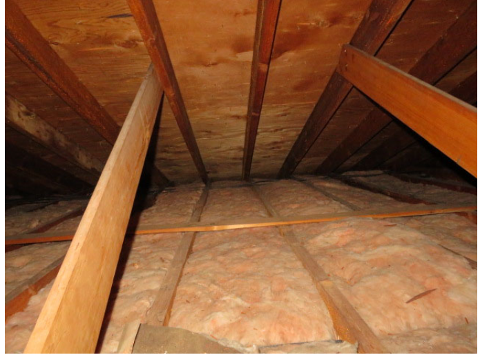
Eave vents. It is recommended the insulation be pulled back from the eave vents to improve the ventilation of the attic.
